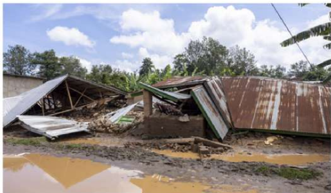
AAR Photo: Flood and and landslides of May 2023 affected communities in Western Province
